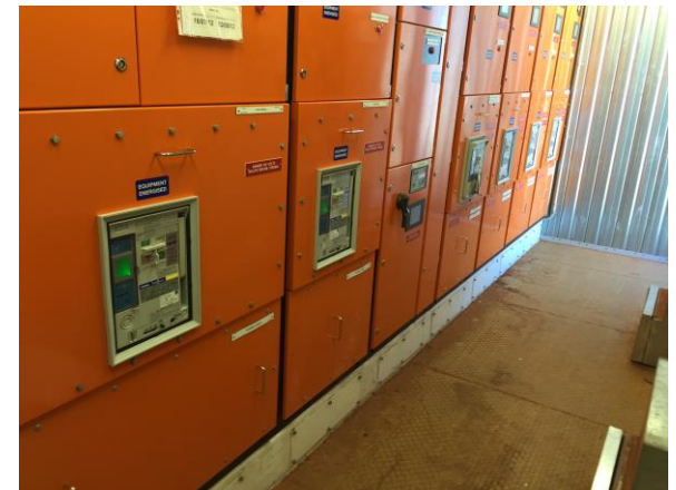
Switchboard with Terasaki equipment at Jimblebar Mine
