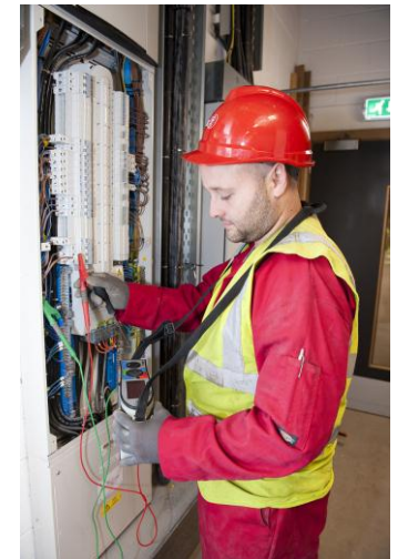
Forth Electrical Services commissioning a Terasaki Pro-DB distribution board in the Arena
