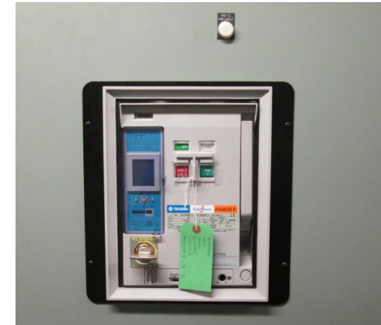
After: Retrofit ACB, protection relay with LCD
