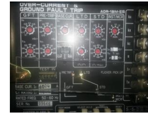
Before: Obsolete protection relay
