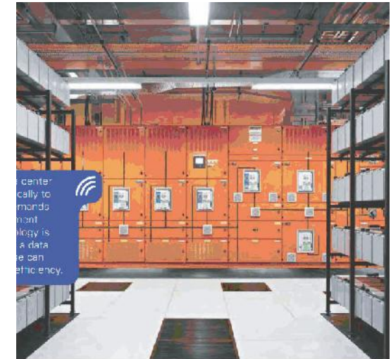
Terasaki ACBs protecting the data load at Telehouse Docklands
